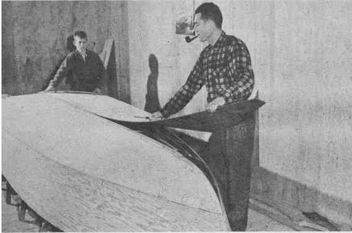
Fitting the last bottom panel in place preparatory to fastening. This father-son team has done a careful job of countersinking all screws.
