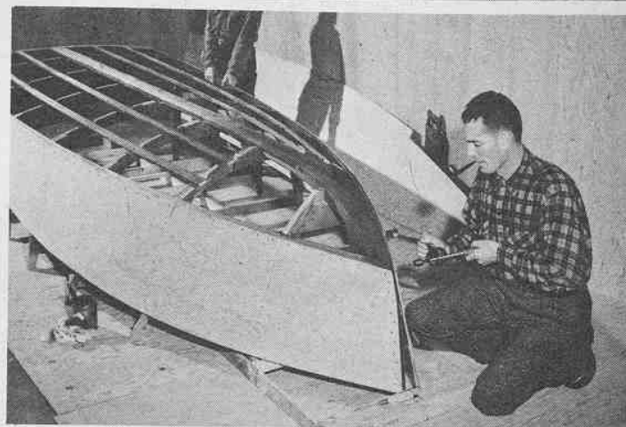
Drilling holes for planking screws is made easier if you have a small electric drill, but it can be done by hand. (Photos continued—See Over)
