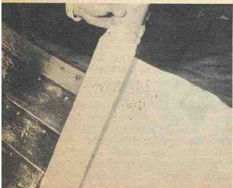
Immediately after the second, or "wet" coat of resin has been applied, a narrow length of cloth is neatly rolled on.
