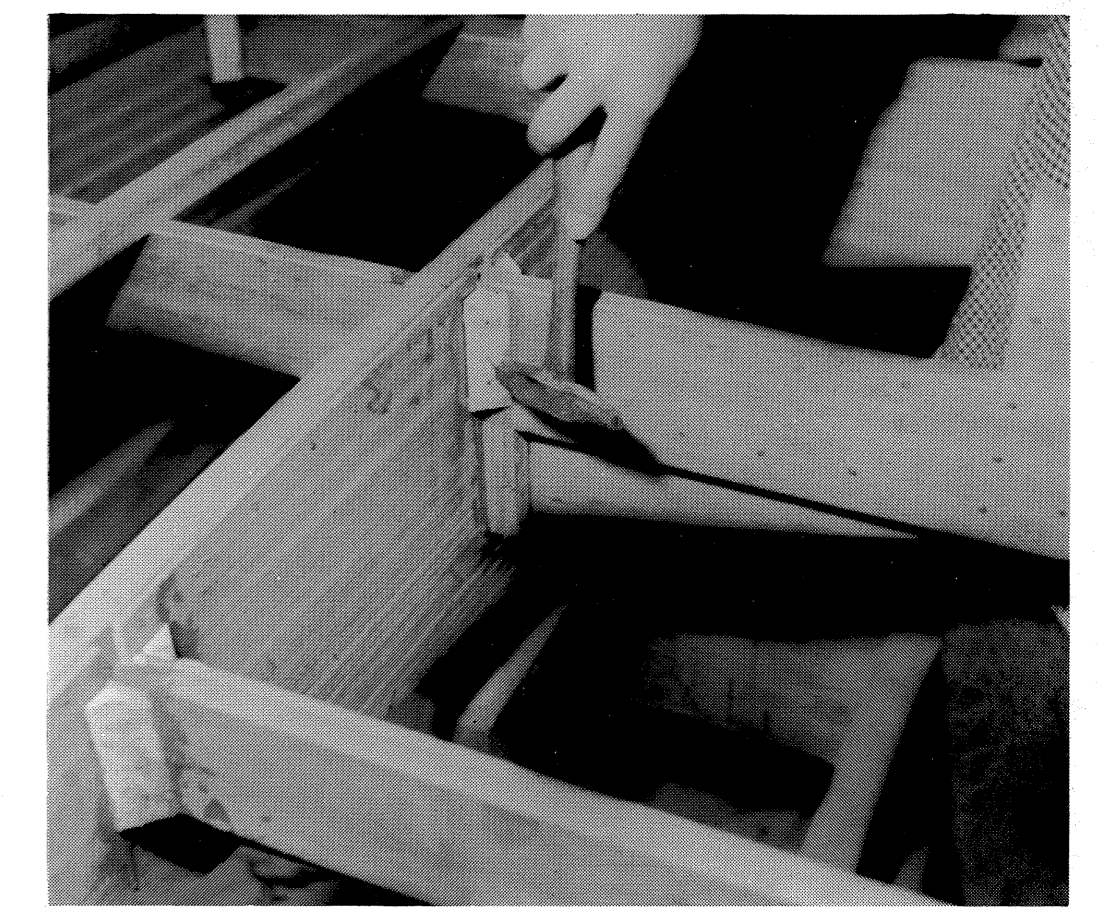
6. Glue blocks are used to fasten all ribs to the girders. 1" wire brads are used.
